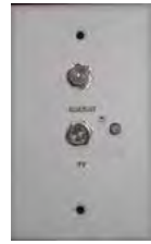
Antenna Power Supply
