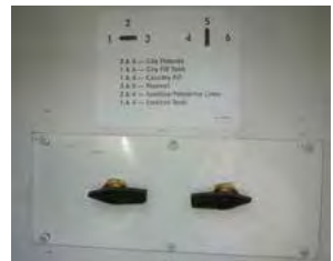
Fig. A -Water Valve Controls
