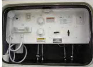
Fig. B - Utility Center
